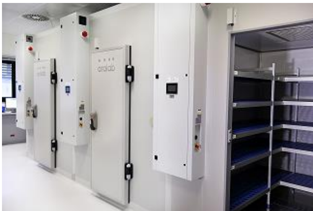
Stability rooms turnkey project by Aralab
